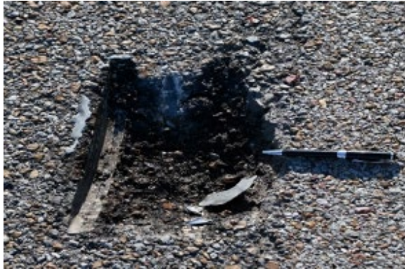
Figure 15 - Pavement Condition After Removal of Snow Plowable Marker
