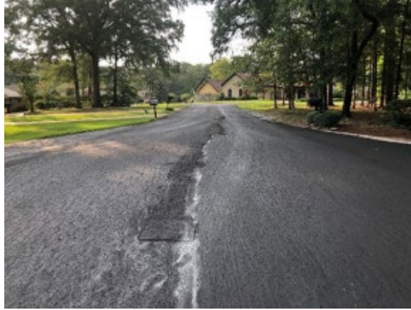
Figure 65 - Unacceptable Longitudinal Joint
