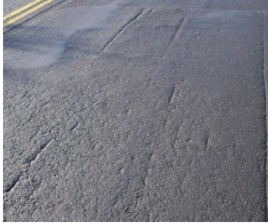
Figure 64 - Excessive Drag Marks and Scratches
