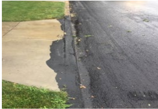
Figure 60 - Poor Workmanship Resulting in Slurry Surfacing on Gutter/Driveway
