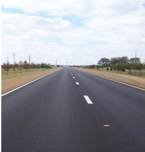
Figure 38 - Acceptable Longitudinal Joint
