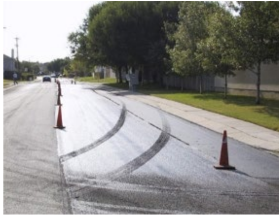
Figure 69 - Damage from Early Traffic
