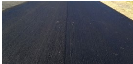
Figure 52 - Lack of Surface Texture Uniformity
