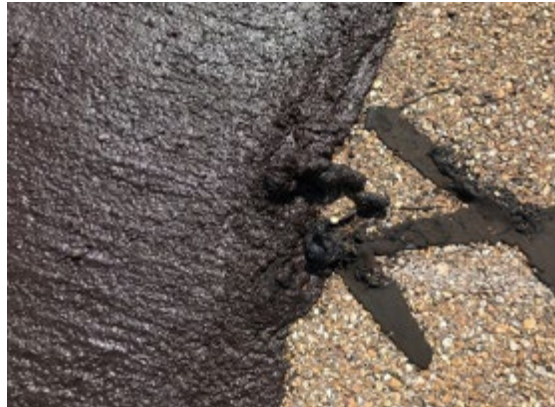
Figure 56 - Excessive Crack Sealant Application
