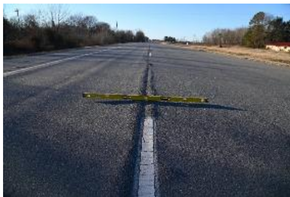
Figure 24 - Unacceptable Candidate for Rut Filling
