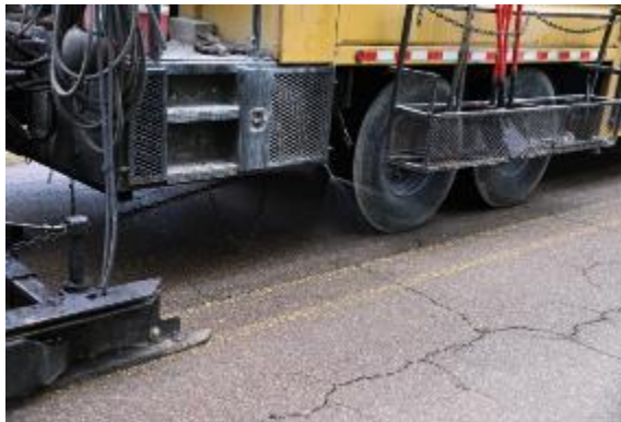
Figure 19 - Water Spray Bar
