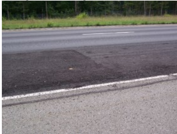
Figure 41 - Unacceptable Transverse Joint
