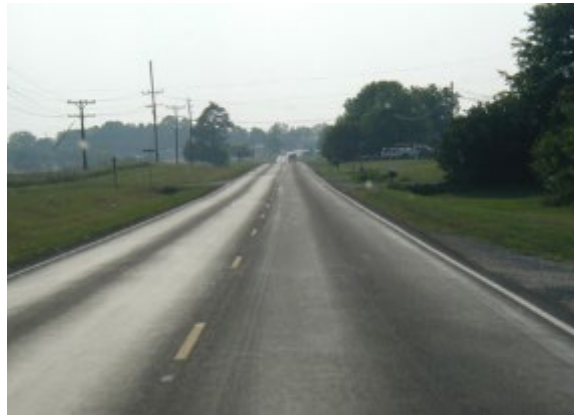
Figure 68 - Flushing Due to Premature Release to Traffic
