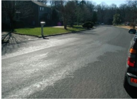
Figure 40 - Unacceptable Transverse Joint
