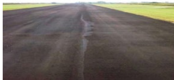
Figure 39 - Unacceptable Longitudinal Joint
