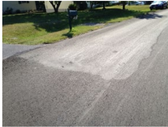
Figure 66 - Unacceptable Transverse Joint (Overworked)
