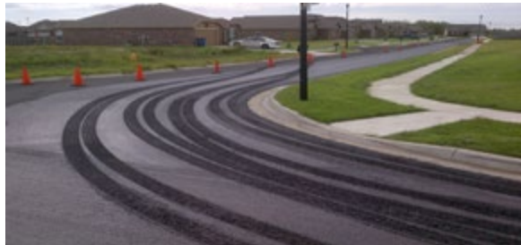
Figure 46 - Damage Due to Premature Traffic – Requires Repair
